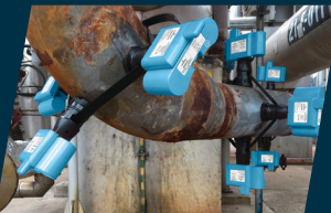
Corrosion Erosion Monitoring
