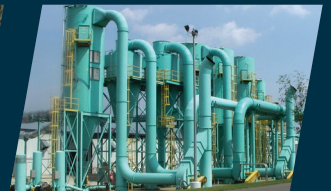
Pneumatic Systems & Process Piping
