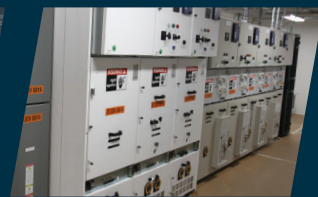
UL 508A & UL 698A Panel Fabrication
