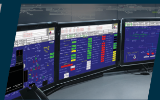
SCADA, PLC, & HMI Design/Programming
