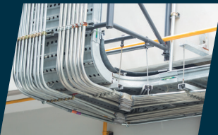
Complete Electrical Installation
