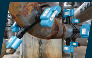
Corrosion Erosion Monitoring
