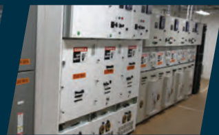
UL 508A & UL 698A Panel Fabrication
