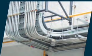
Complete Electrical Installation
