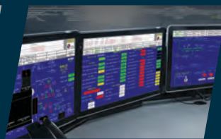
SCADA, PLC, & HMI Design/Programming
