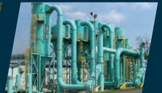
Pneumatic Systems & Process Piping
